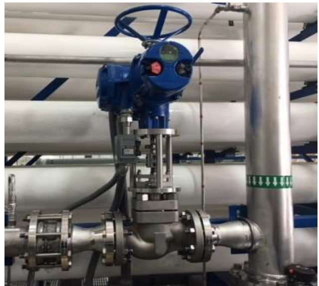
New installed valve on train #1
