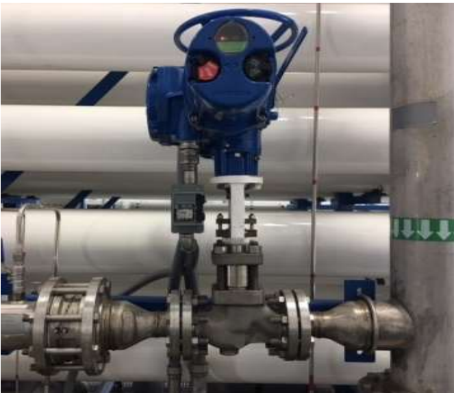
Old concentrate valve on train #1
